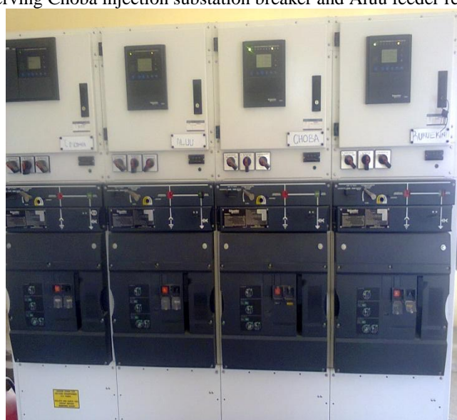
Fig 2: Choba injection substation breaker
