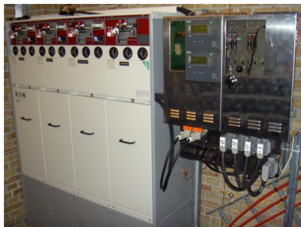
Fig. 11 First online SACSe station
