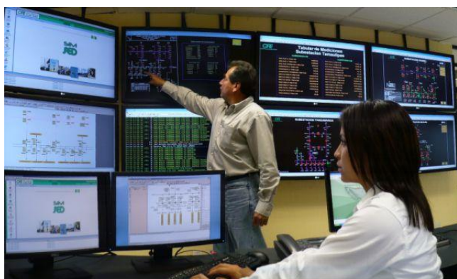
Fig. 6. On-Line Simulator installed in Monitoring and Analysis Center at Division Golfo Centro.
